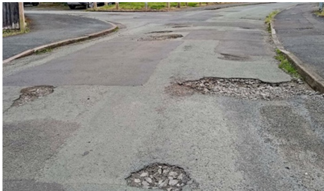
A Cleveland street in need of repair. Credit: YouTube.
